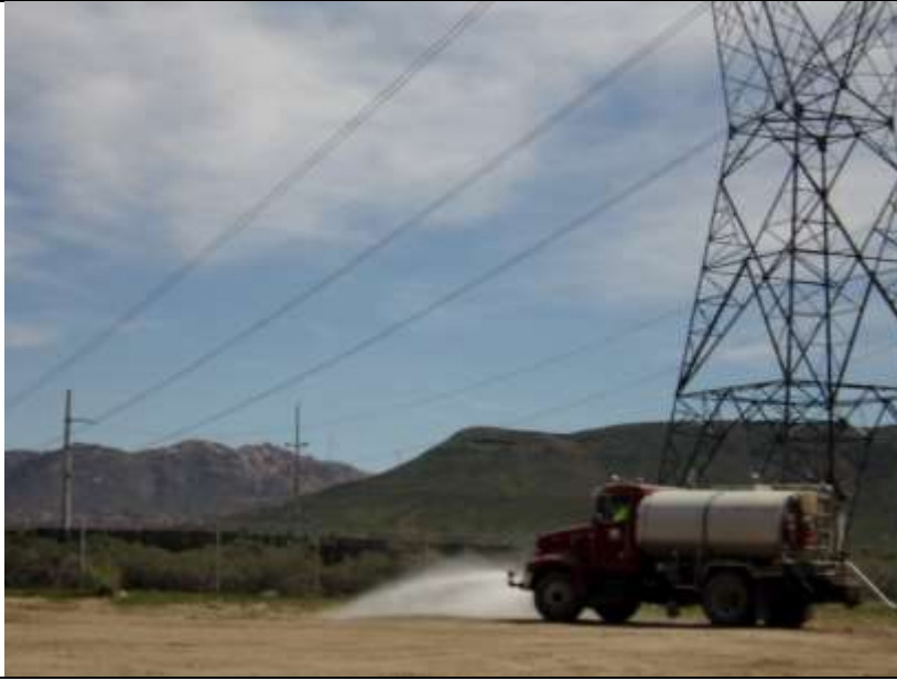
Photo 3: Water trucks were present to suppress dust emissions during restoration work in compliance with MM-BIO-4a and MM-AQ-1.
