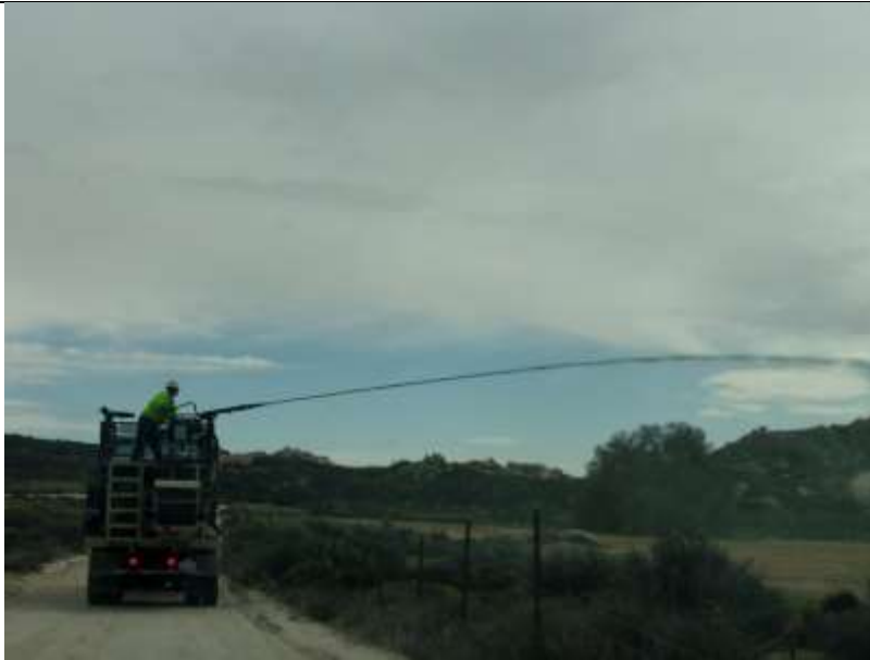
Photo 1: In accordance with the Habitat Restoration Plan and MM-BIO-1d, crews completed clean-up and restoration of the Jewel Valley staging area. All construction materials and debris were removed and temporary work areas were hydro-seeded with native seed mix.
