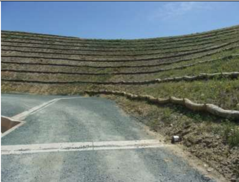
Photo 2: Drainages and erosion control devices along the ROW were in good condition according to the Project SWPPP and MM-HYD-1.
